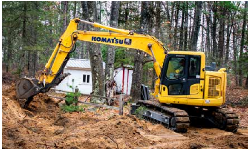
Curtis Excavating operator Andy Curtis moves dirt with a Komatsu PC138USLC tight tail swing excavator.
