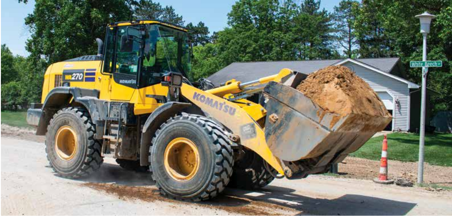
An American Excavating operator moves dirt with a Komatsu WA270-8 wheel loader on a utility project in Saginaw, Mich.
